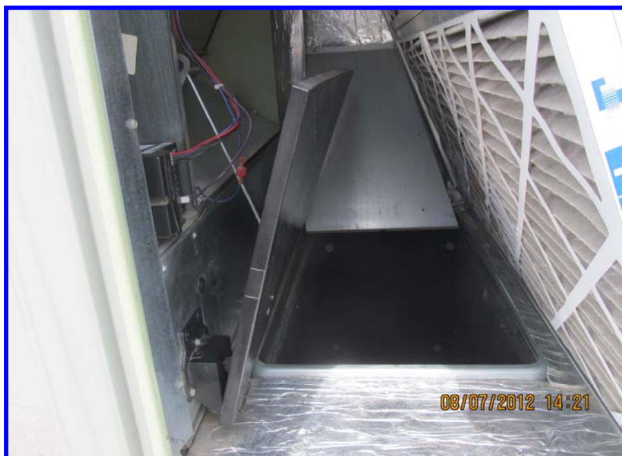
ROOM # 101-AHU - RETURN AIR-PLENUM
