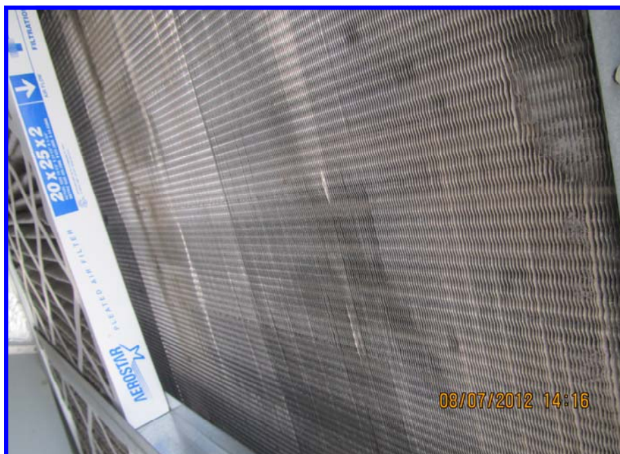
ROOM # 104-AHU - COOLING COIL
