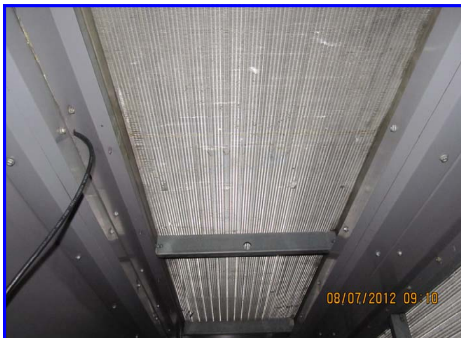
AHU # 6-HEATING COIL-DOWNSTREAM
