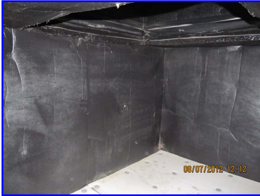
AHU # 2-RETURN AIR-PLENUM
