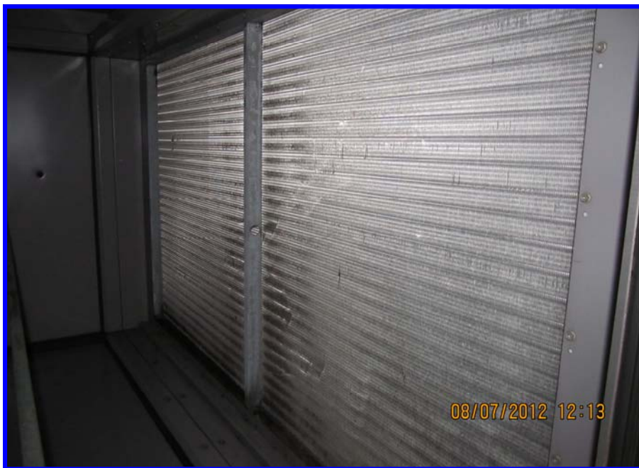
AHU # 2-COOLING COIL-UPSTREAM
