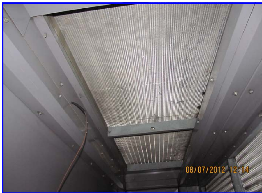
AHU # 2-HEATING COIL-DOWNSTREAM
