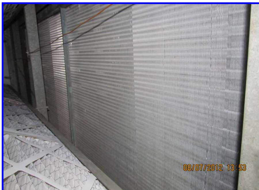
AHU # 10-RETURN AIR-PLENUM
