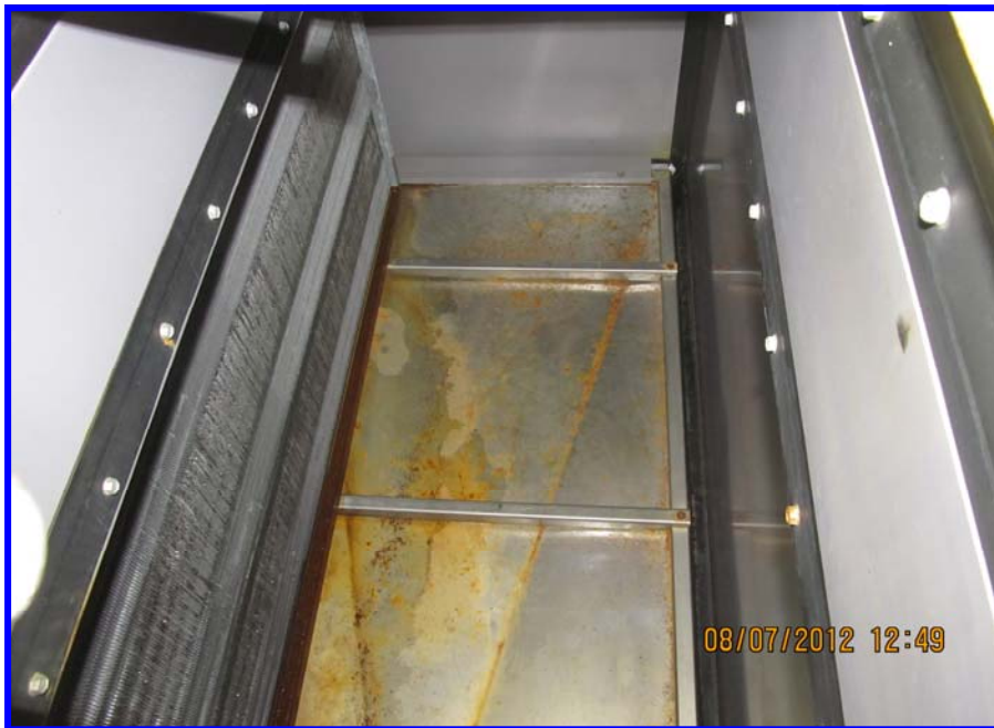
AHU # 1-DRAIN PAN
