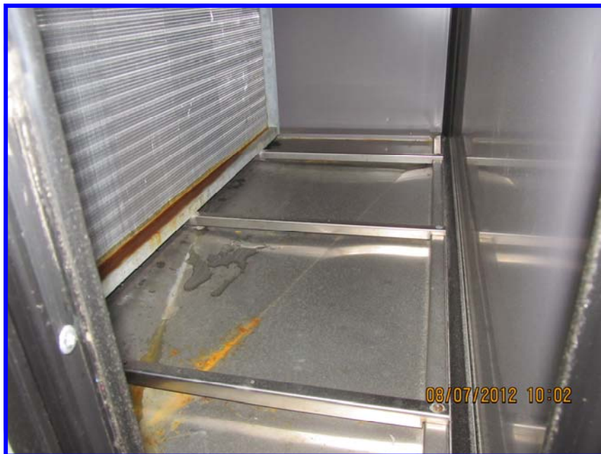
AHU # 5-DRAIN PAN
