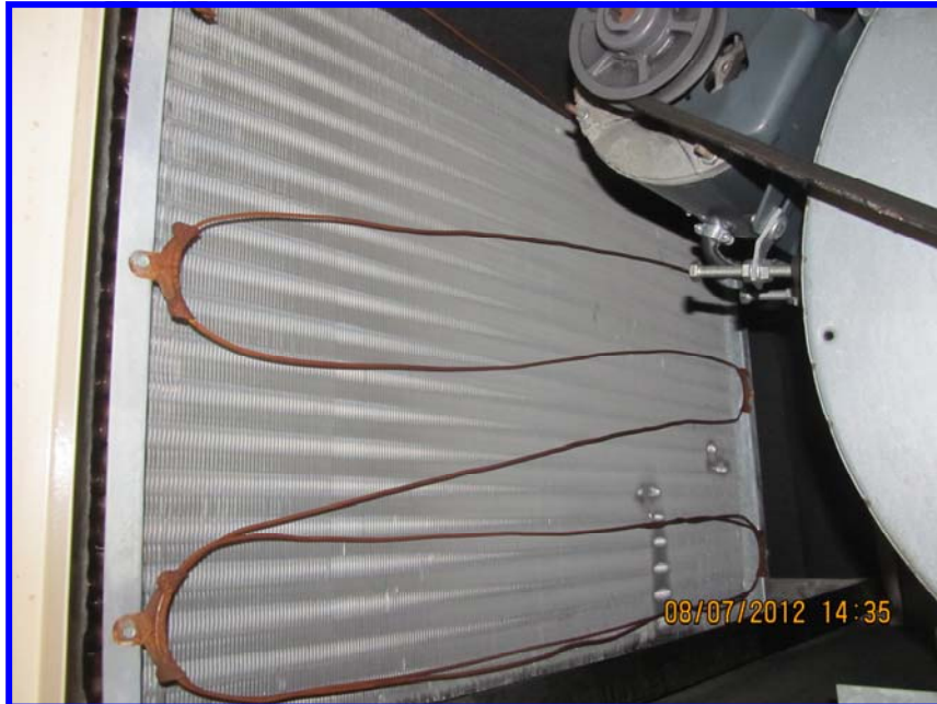
ROOM # 400-AHU-COOLING COIL
