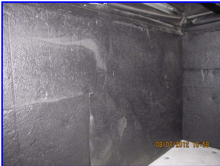
AHU # 3-RETURN AIR-PLENUM
