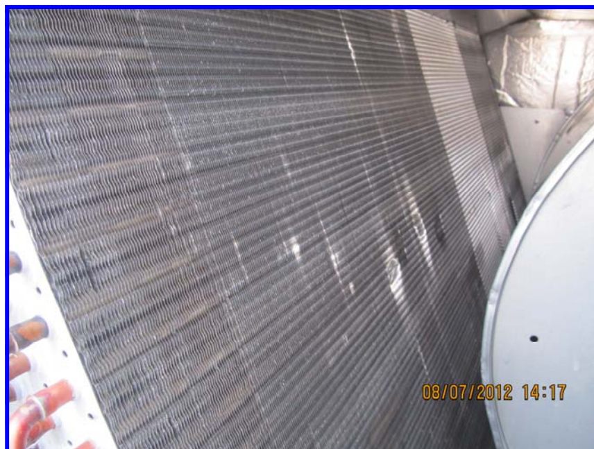
ROOM # 104-AHU-HEATING COIL
