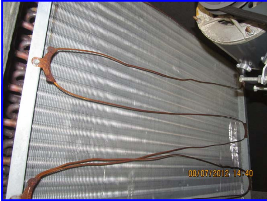
ROOM # 405-AHU-COOLING COIL
