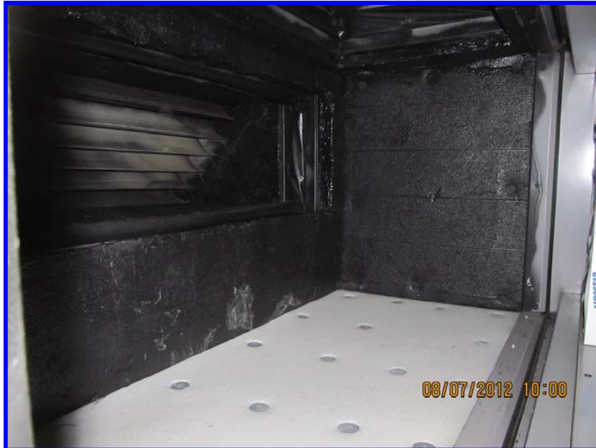
AHU # 5-RETURN AIR -MIXING PLENUM
