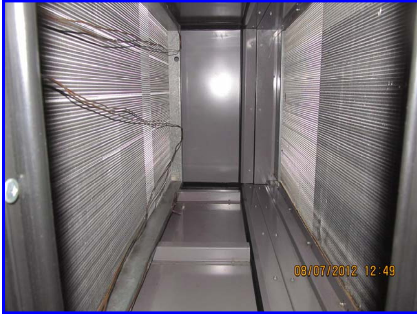
AHU # 1-COOLING COIL
