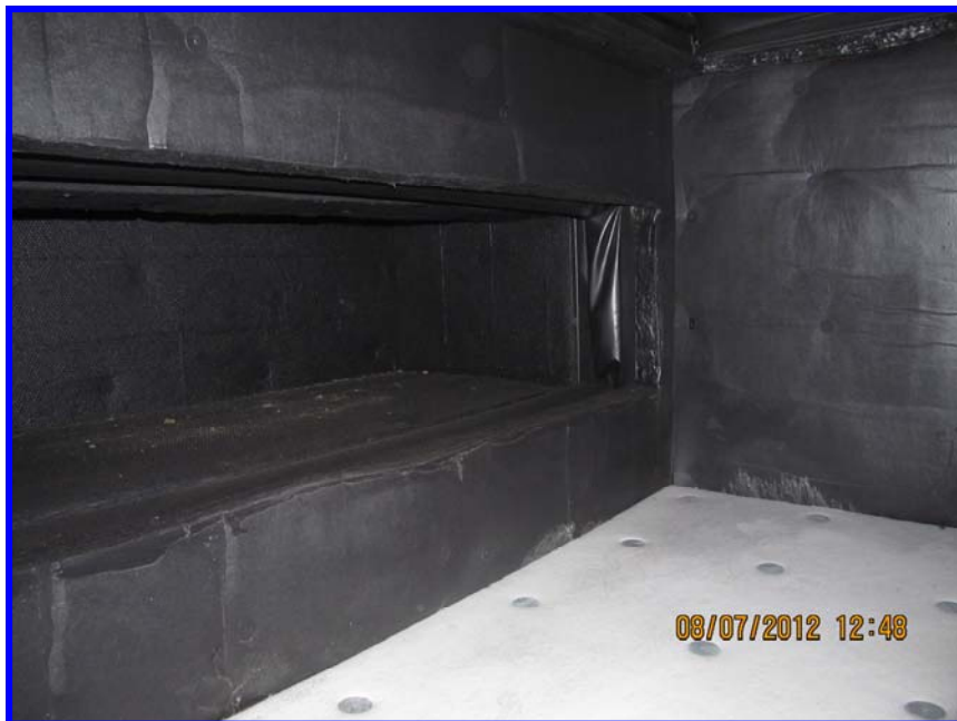
AHU # 1-RETURN AIR-PLENUM
