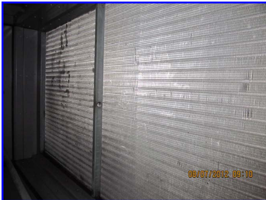
AHU # 6-COOLING COIL-UPSTREAM
