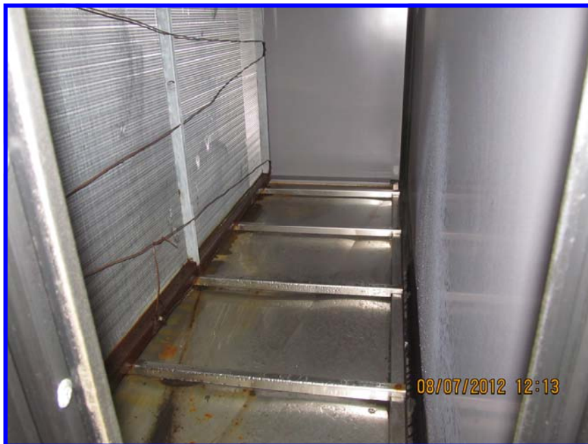
AHU # 2-DRAIN PAN-COOLING COIL-DOWNSTREAM
