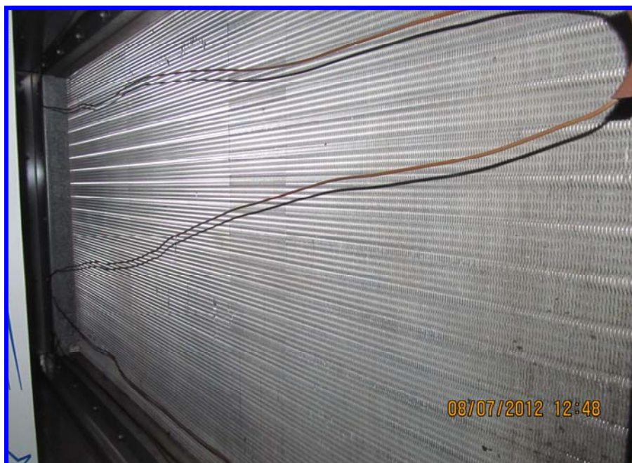
AHU # 1-HEATING COIL-UPSTREAM
