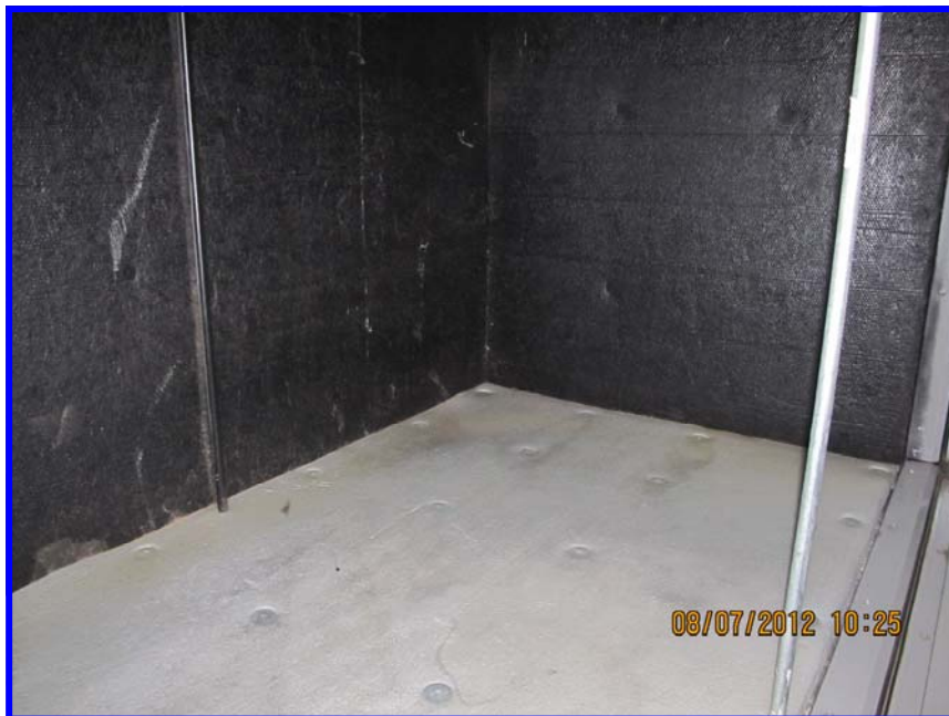
AHU # 4-RETURN AIR-PLENUM
