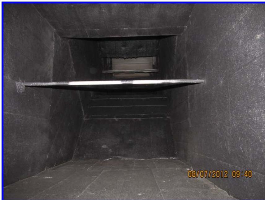
AHU # 6-RETURN AIR DUCT UP FROM UNIT
