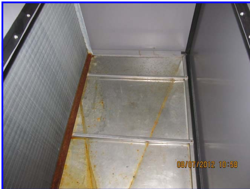
AHU # 3-DRAIN PAN/COIL-DOWNSTREAM
