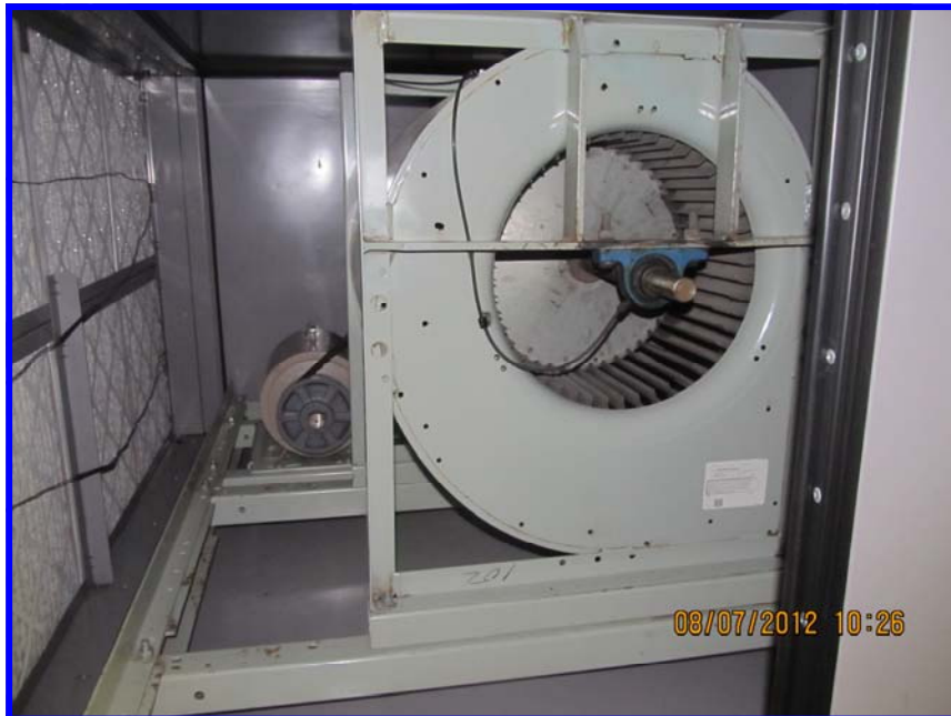
AHU # 4-BLOWER COMPARTMENT
