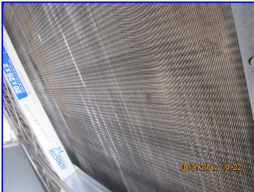
ROOM # 101-AHU-COOLING COIL
