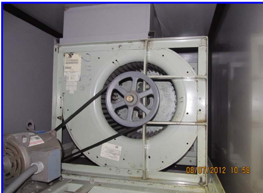
AHU # 3-BLOWER COMPARTMENT
