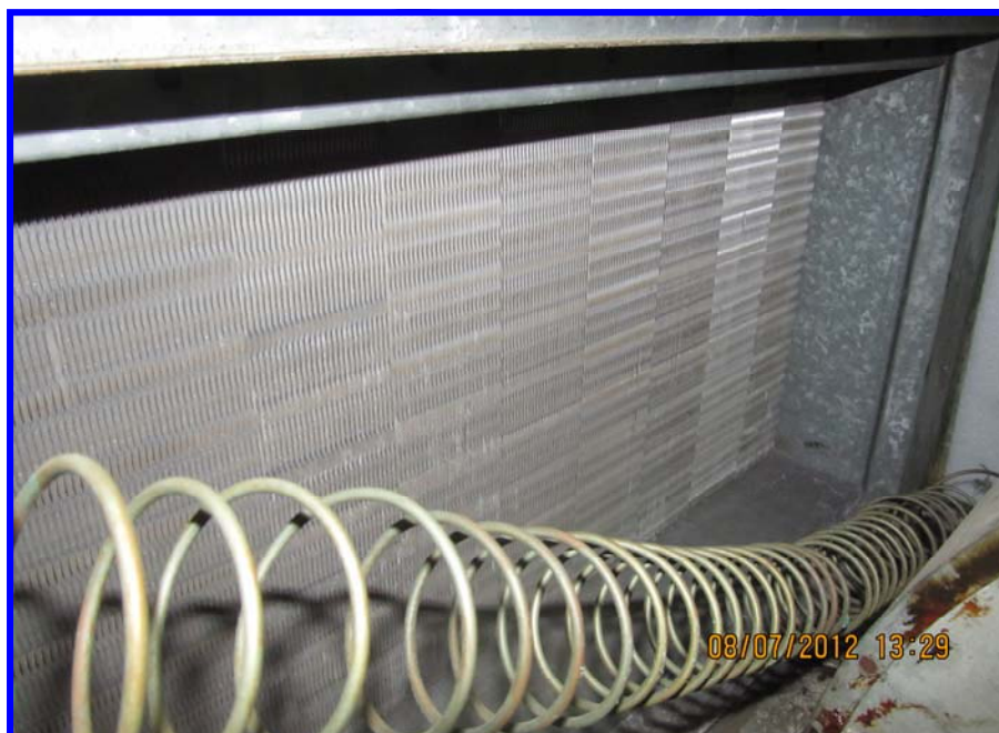
AHU # 8-COIL-DOWN STREAM
