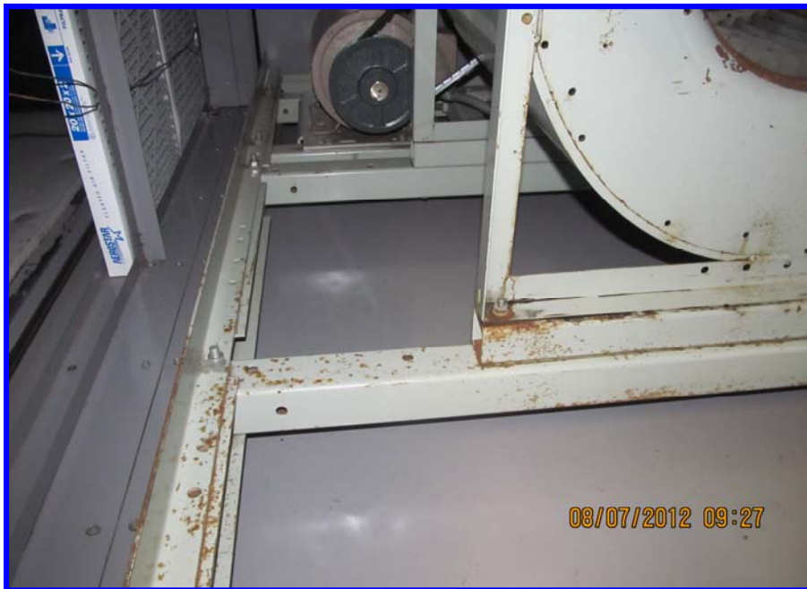
AHU # 6-BLOWER COMPARTMENT-FLOOR
