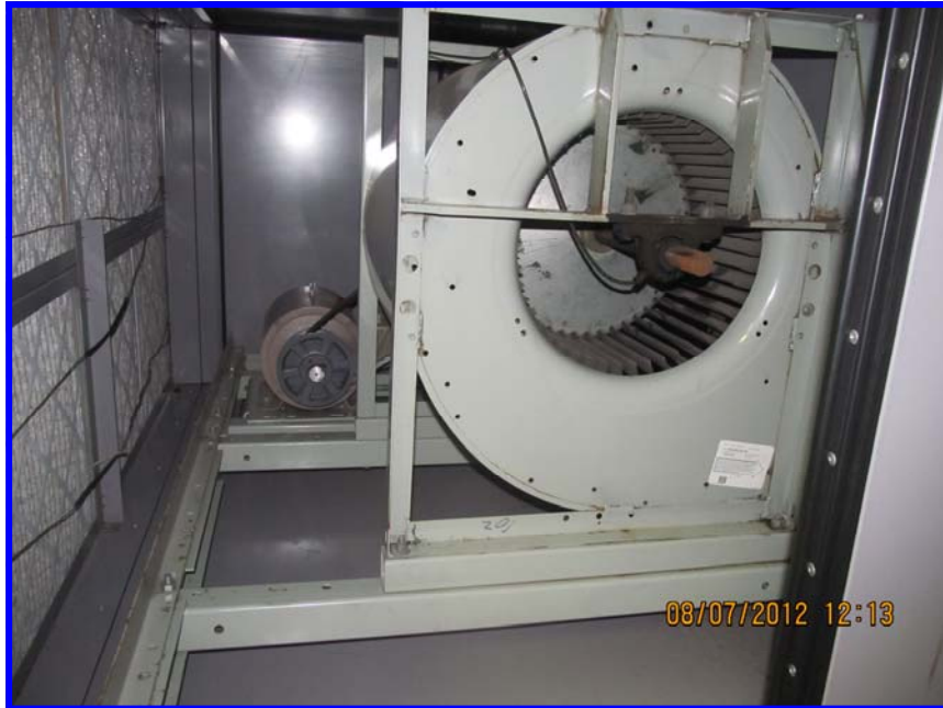
AHU # 2-BLOWER COMPARTMENT
