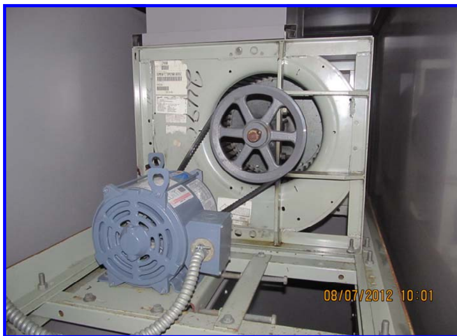
AHU # 5-BLOWER COMPARTMENT
