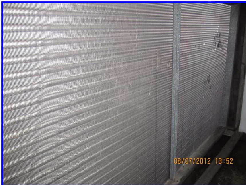
AHU # 10-COOLING COIL
