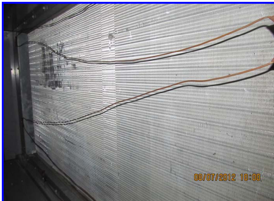
AHU # 5-HEATING COIL-UPSTREAM
