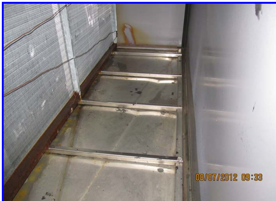
AHU # 6-DRAIN PAN
