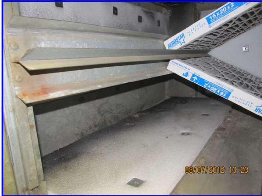
AHU # 8-RETURN AIR-PLENUM
