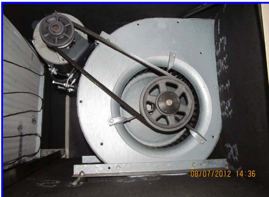
ROOM # 400-AHU - BLOWER
