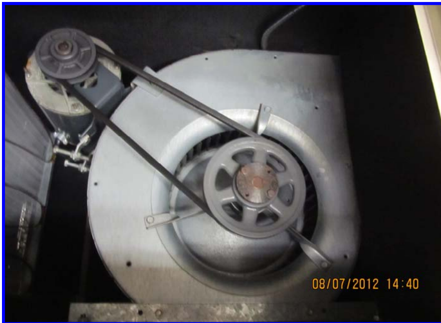
ROOM # 405-AHU - BLOWER
